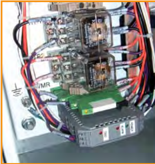
Small Orion-based RTU panel with optional 48V dc NovaTech Battery Monitor
