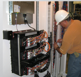
On-site at DC-area substation
