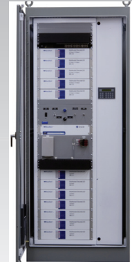
RTU Panel with Orions and DDIOs
