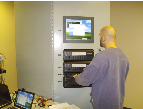
NovaTech software engineer Brock Haas checking out the RTU HMI in Lenexa, KS prior to factory acceptance test. NovaTech was responsible for procurement, assembly and screen engineering of the industrial PC-based HMI.
