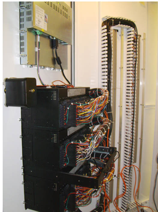
Inside rear view of RTU panel assembly showing network connections and wiring to HMI PC, Automation Controllers and supy/local control switch.
